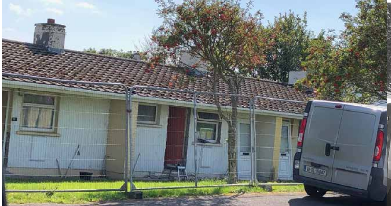
Work Beginning on the Demolition of Senior Citizens Houses on the Chapel Road in Dunfanaghy. The houses were built in the 1970's and were in use until a few years ago and are now to be replaced by more modern buildings. This work has been welcomed by local Cllr Michael McClafferty who says "there is much need in the local area for housing needs and good luck to the appointed contractor".
