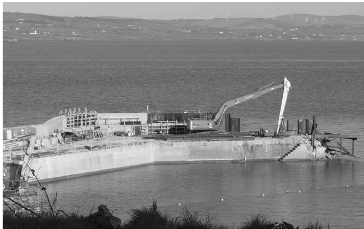
Race against time... with the new deadline of the end of April 2024 for the completion of works at Portsalon Pier, the job seems far from complete and according to sources it will also miss the June Bank Holiday as well. Progress on the pier has been extremely slow and all previous deadlines including Halloween, Christmas, Easter and April all missed.
