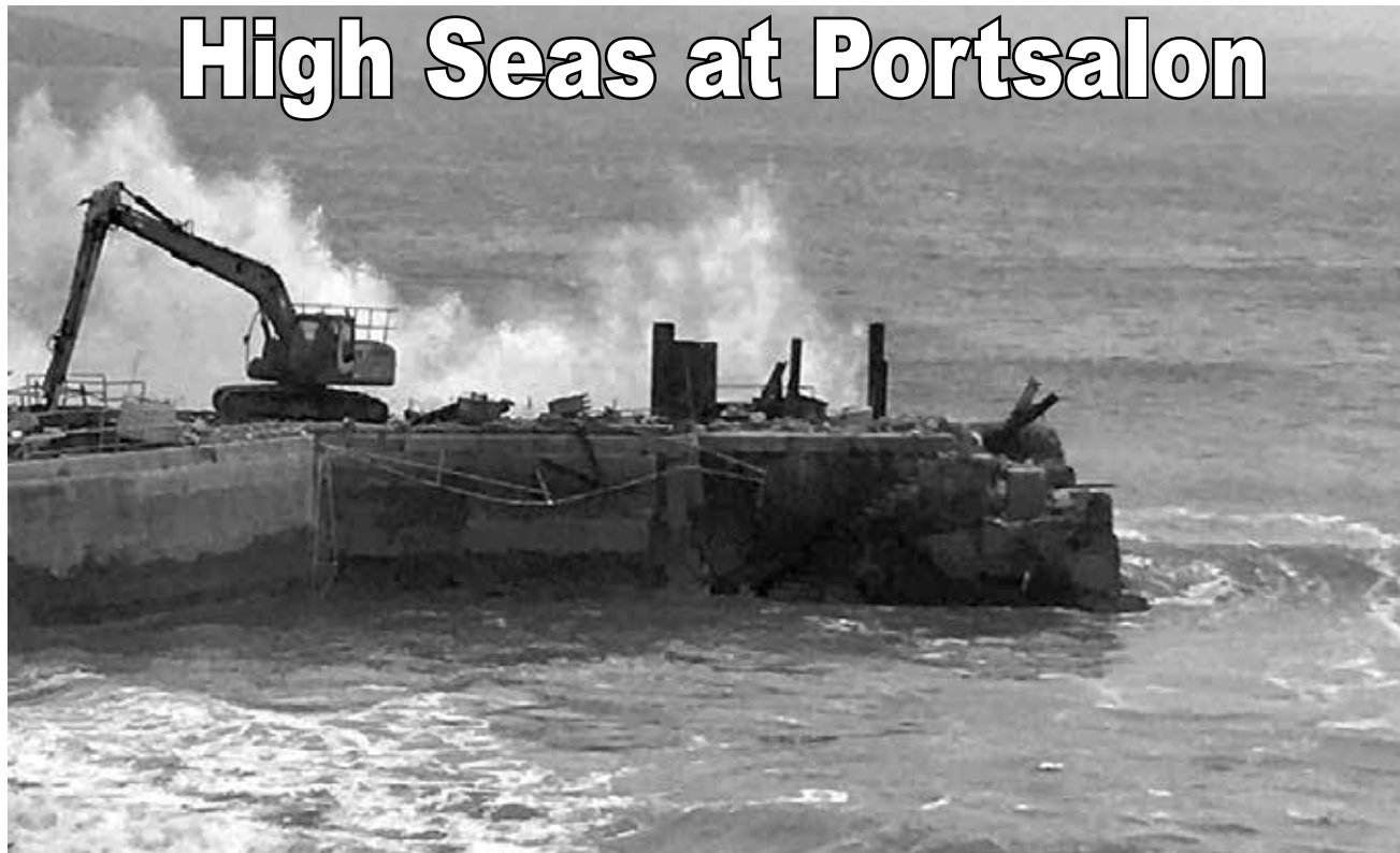
Gale force winds and high seas damaged the ongoing construction work on Friday afternoon when workers were forced to abandon the scene. The dramatic picture was captured by Mary Doherty who had been swimming nearby.
