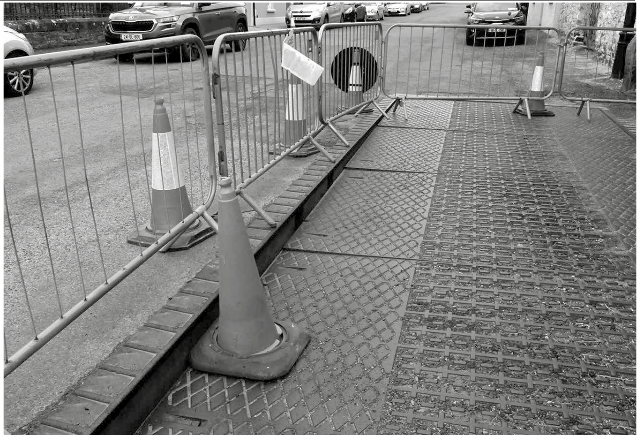
Historic weighbridge sinks.... The old Avery Weighbridge opposite the Town Hall in Ramelton has sank by as much as 6inches in the past week. Cllr. Paucic McGarvey has pointed to the location being used extensively for car parking and has called on the Council to take appropriate action. In the meantime the area is cordoned off for safety.
