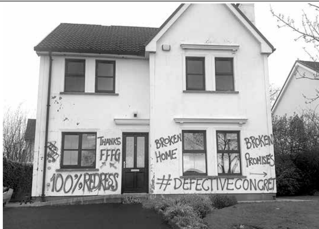
Graffiti sprayed on a house at Coylin Court in Ramelton showing the frustration with the defective concrete campaign.
