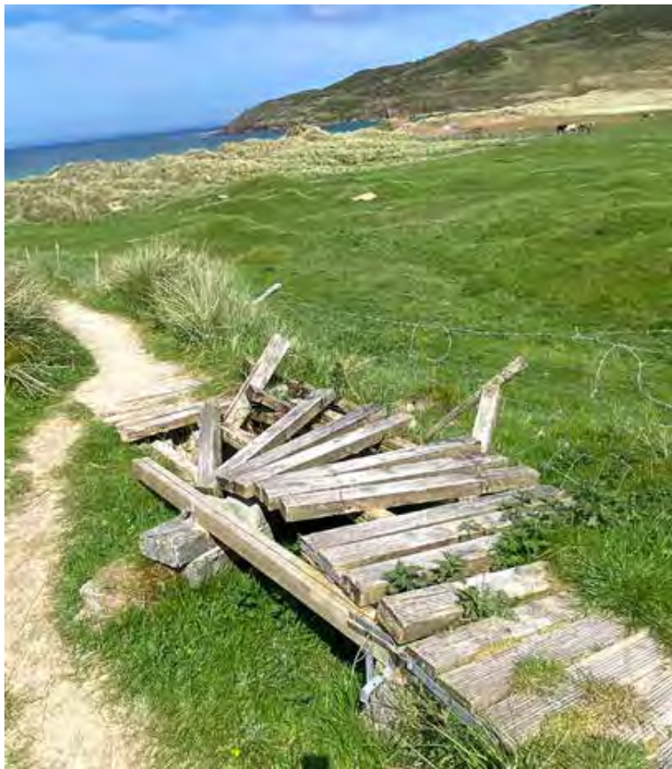
The damaged boardwalk at Trá na Rossan.
