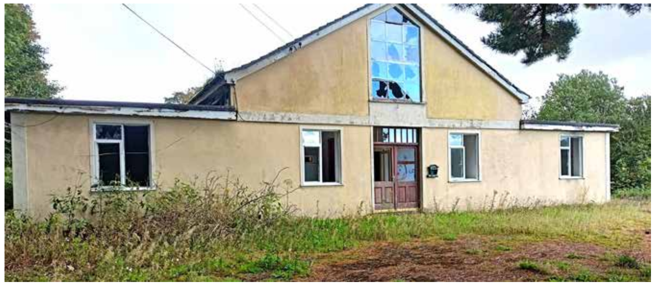
The outside view of the derelict Colaiste Uladh building which is in a state of disrepair.
