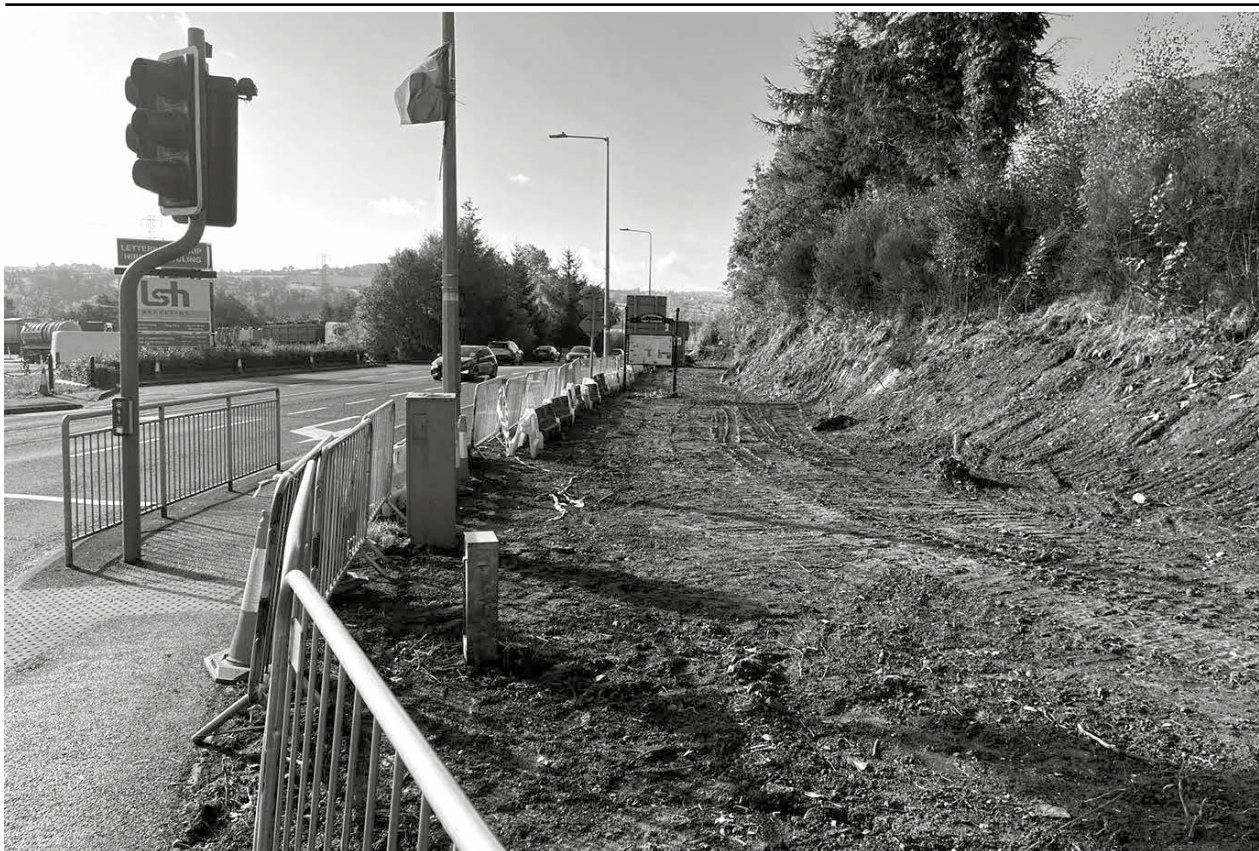
Works continuing on the Ramelton Road and Ballyraine on an Active Travel project that will see the construction of a new cycle lane and upgraded pedestrian footpaths from the old Creamery Roundabout to the Polestar junction
