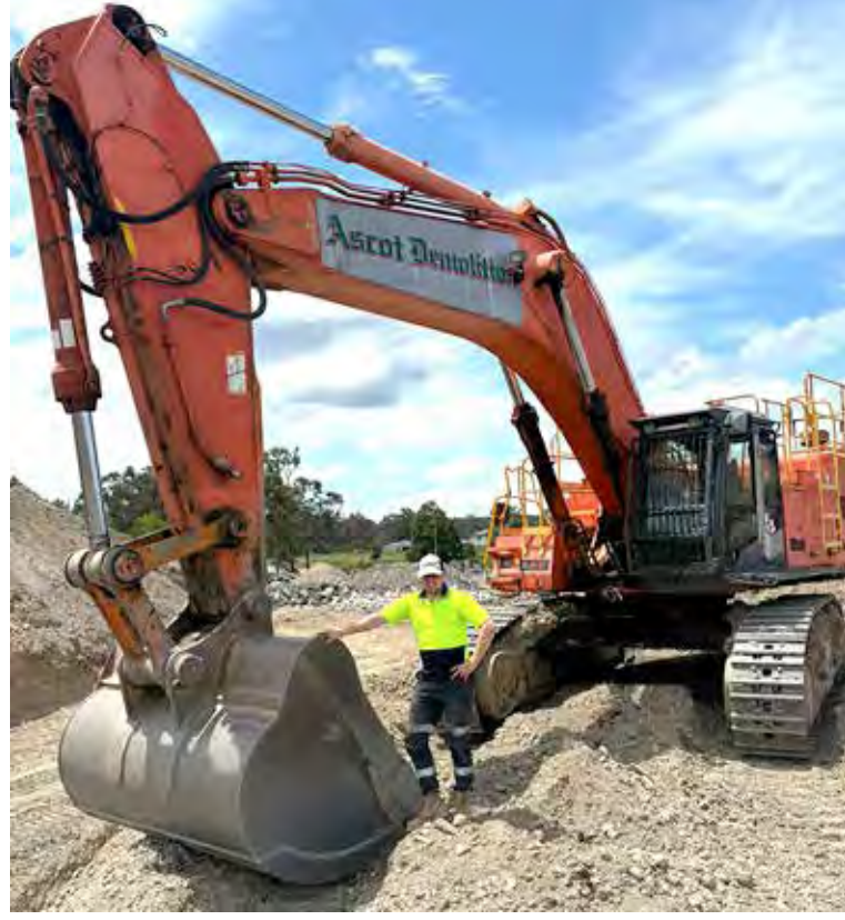
Fionn Woods from Gort a' Choice posing with his seventy-ton track machine while working on a site planned for massive shopping and housing in Logan. The site has Irish workers from every county and parish in Ireland.
